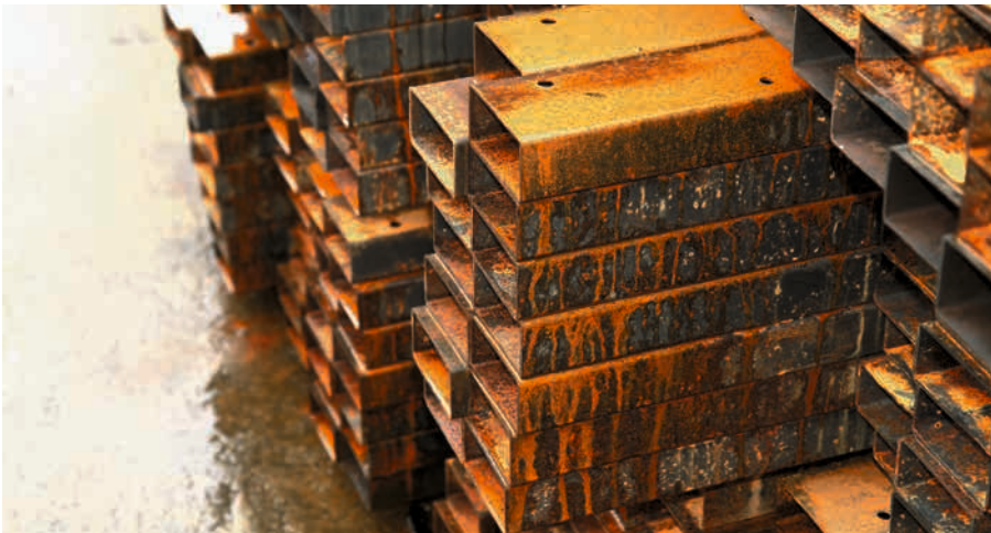
Fig. 4: Corrosion of steel components.
