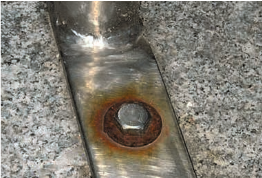
Fig. 12: This is a typical case of contact corrosion. A zinc-plated carbon steel (washer) and stainless steel (screw and part) were used together. The surface area of the more noble metal – the stainless steel – is larger, causing strong corrosion of the washer.
